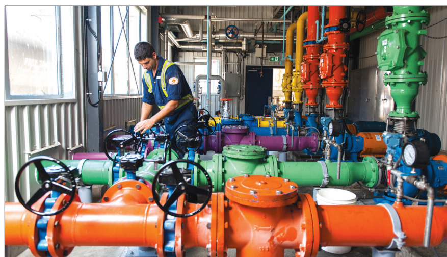
“These colour coded pipes are used to pump canola oil and tallow at West Coast Reduction’s Port of Vancouver facility.”
